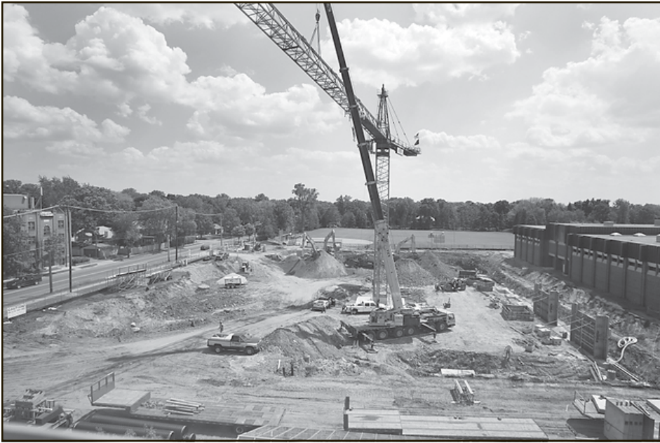
Here's a peek at early excavation of the site for the new ramp, looking south.
