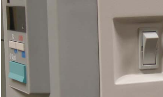
1. Main power on off switch.
